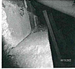
Brick separation on road side.
