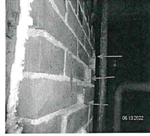
Step crack with horizontal separation of bricks on road side. Recommend a qualified engineering firm conducts a full structural assessment.
