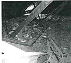
Attic pile of what appears to be slate shingles/ tiles for roof.
