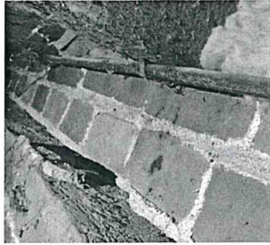
Recommendation: to Have a qualified Engineer to a complete structural assessment of the building from the basement to the roof.
