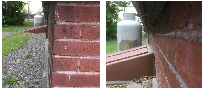
Bulkhead side sweep in foundation wall. Recommend a qualified engineering company do a complete structural assessment of the building.
