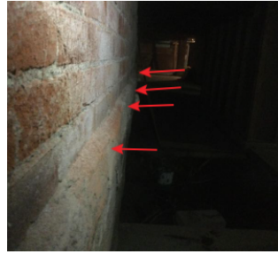
Foundation wall on parking lot side has evident inward bow. Recommend wall is assessed by a qualified engineer and repaired accordingly.
